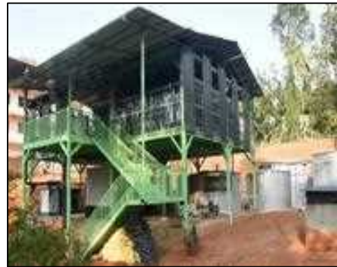
1 MLD STP at Kozhikode medical College
