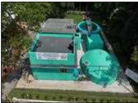
360 KLD STP at General Hospital, Thrissur
