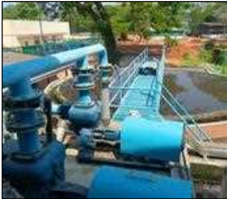
500 KLD STP at Kozhikode medical College
